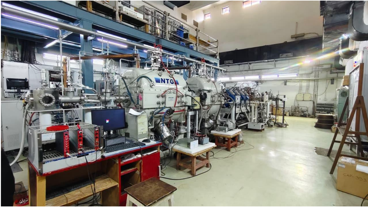
Figure 2. A photograph showing the 4th and 5th heavy-ion linac module L4, L5 in the RIB facility.
